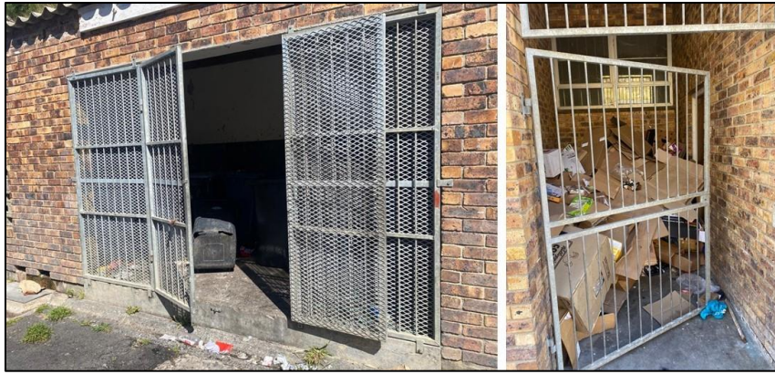
Figure 7. Open waste rooms at Waterfall Barracks.
